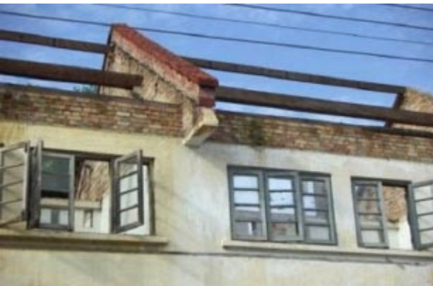
Second floor. Notice the red brick used for construction. They are still in good form.
