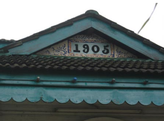
Kampong Kepayang’s Masjid Ahmadiyah, 1905. Note the Chinese influence in the painted decoration. Photo : Mai Palmer.
